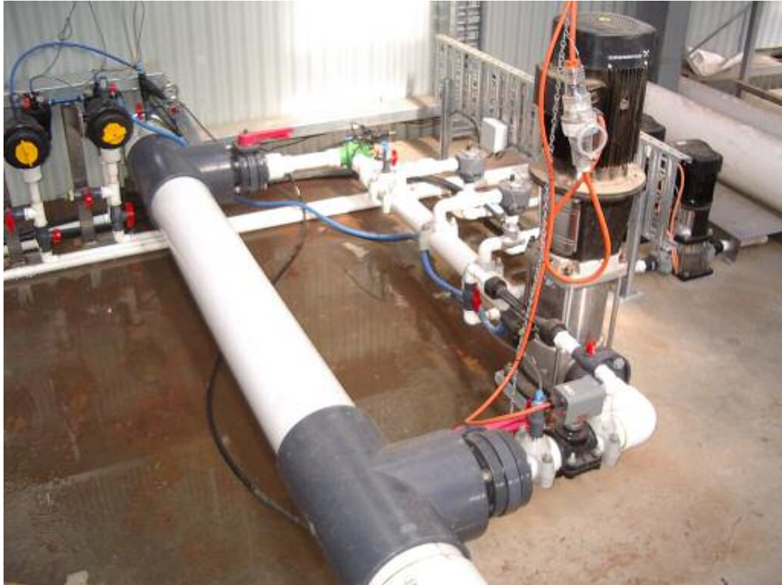
Figure 13: A centrifugal bypass fertigation system used for an OH program
